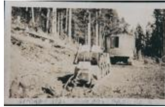
[Photo of gas shovel transporting fuel] (2023_09_01_02_02_015)
